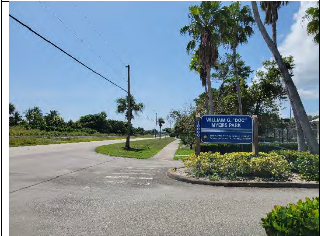
Faded Crosswalk near William 'Doc' Myers Park - South
