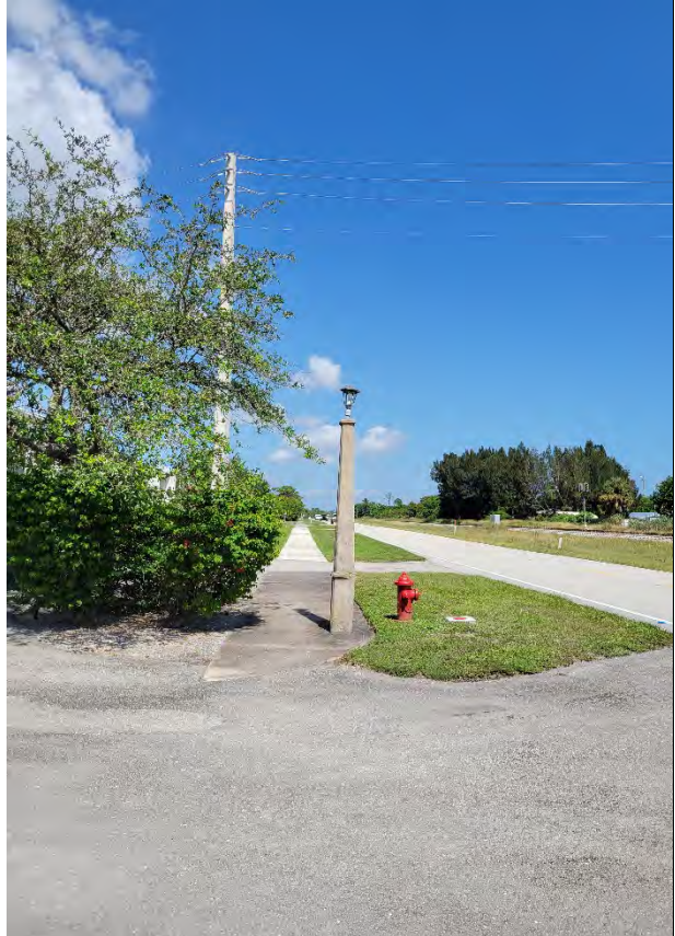
Light Pole Partially Obstructing Sidewalk, Missing Textile Surfaces, adjacent to Wittman Textiles - North
