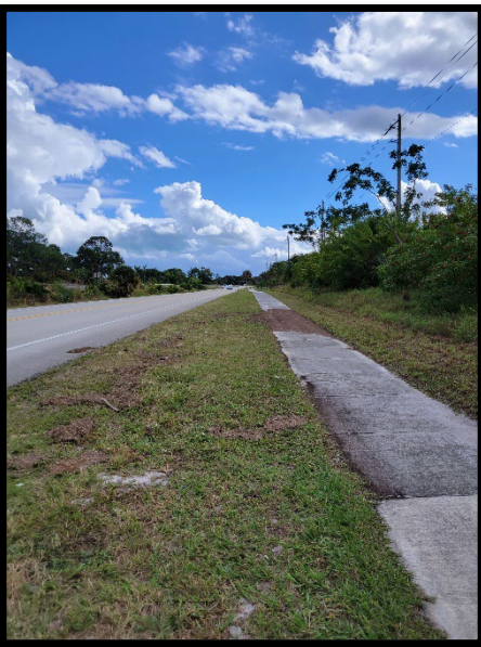
Figure 28: Evidence of Sidewalk Flooding
